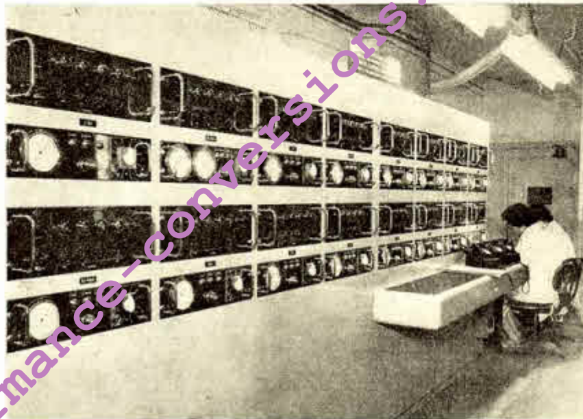
The control panel of the automatic liquid-metering system designed by Automatic Control Engineering Ltd. for General and Industrial Paints Ltd.
