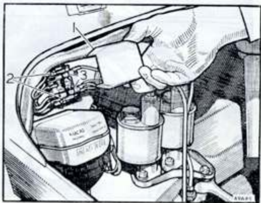
The fuse holder with the plastic cover removed
